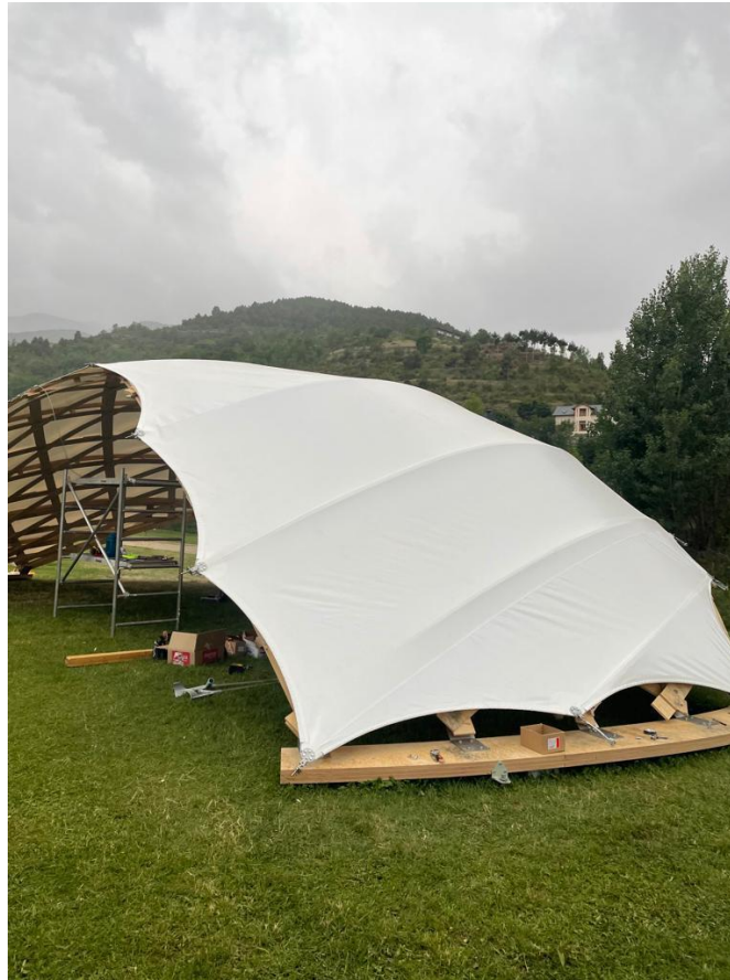
Figure 8. For the manufacture of the PVC membrane, the measurement was obtained through the program and after that it was ordered to be manufactured, which gave it an accuracy to assemble all the screws, tensioners and stainless-steel cables. This promotes digital manufacturing and computational design as a highly competitive and innovative tool. Source: Mauricio Díaz Valdés
